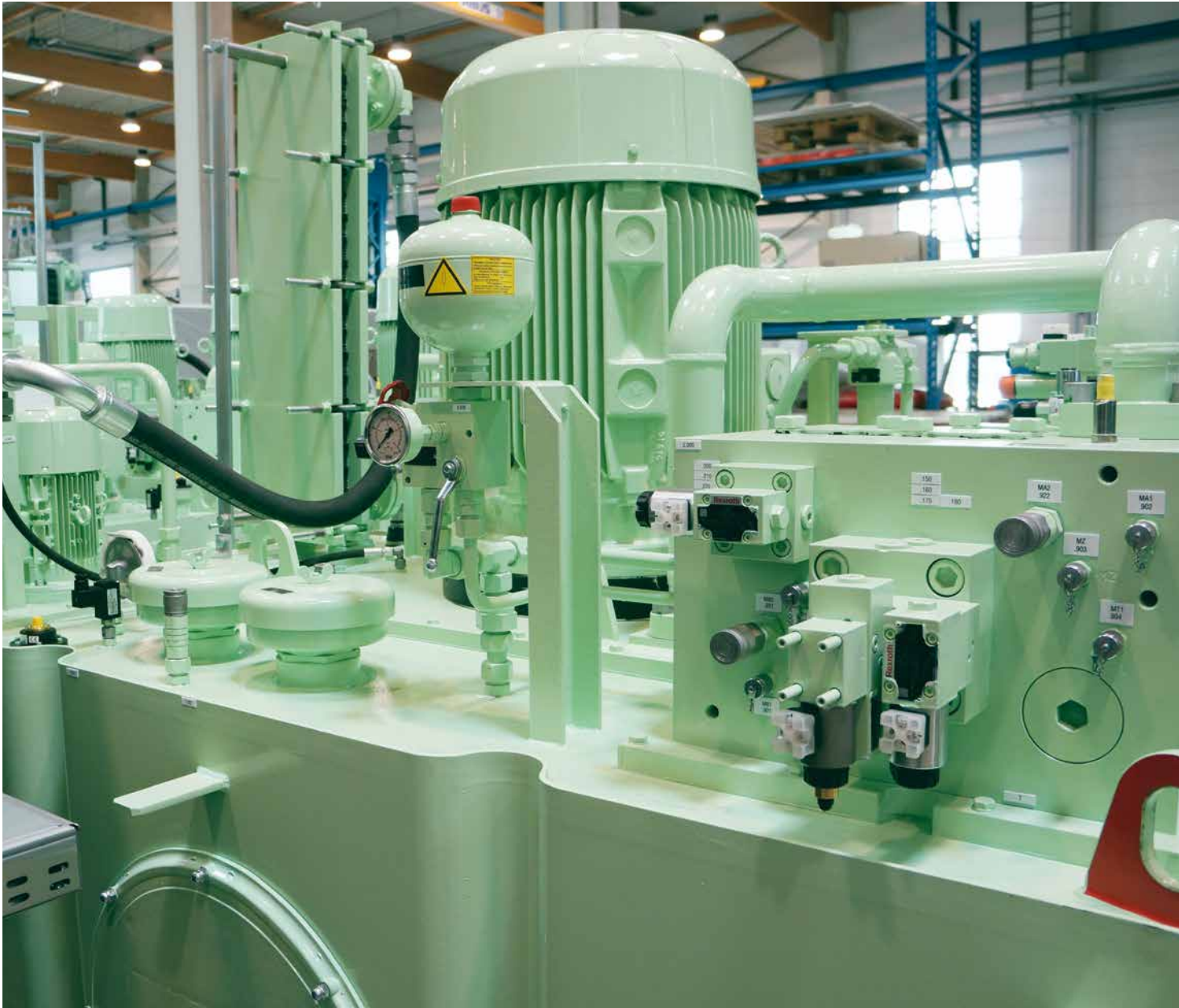
Hydraulic power increase with new installed pumps and advanced hydraulic piping upgrades
